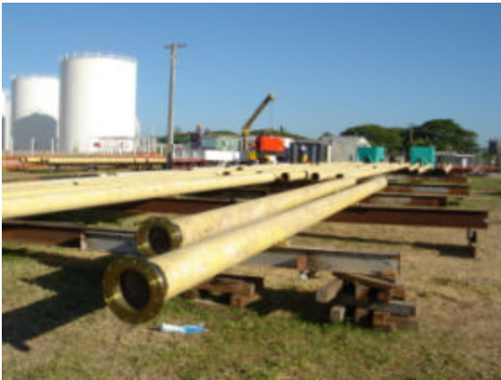
Pipeline Project worksite in Fiji, workers in background are TIG welding a flange in tents
